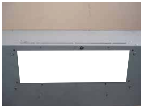
Horizontal Ducting (3-1/4"x10" Rectangular)
